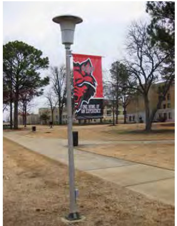
Non-conforming fixture with banner mount attached.
